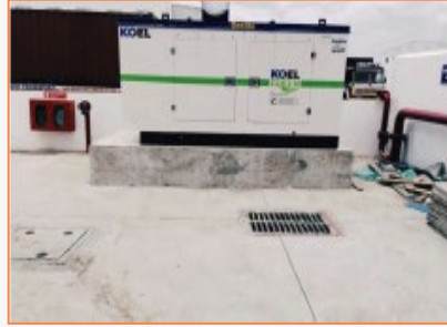
DG Set and Fire Hydrant
