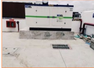
DG Set and Fire Hydrant
